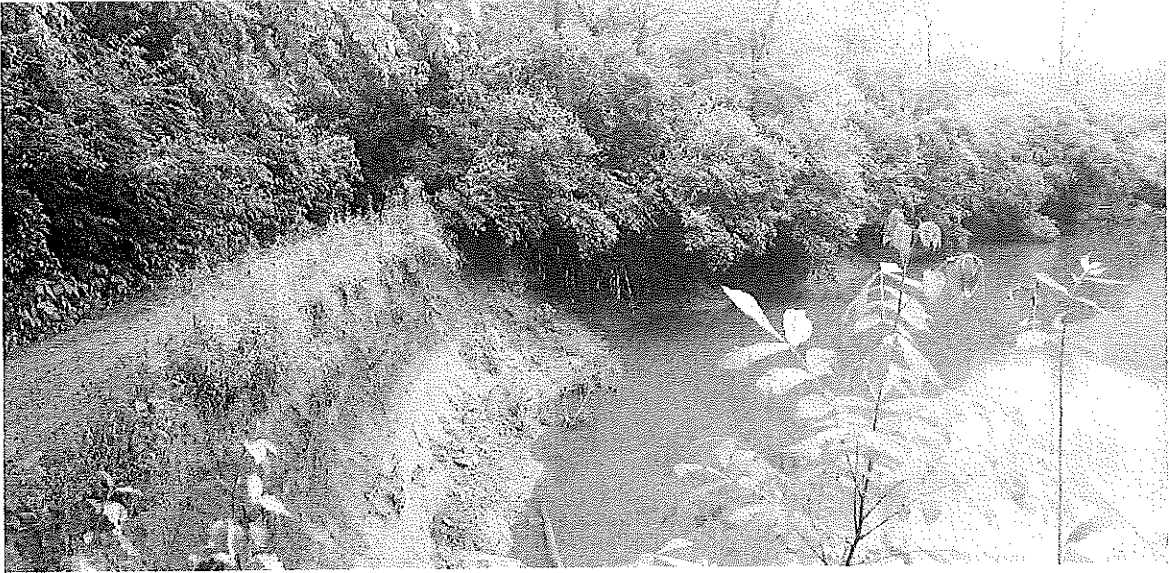
Dick's Creek Erosion – near STA 315+00
