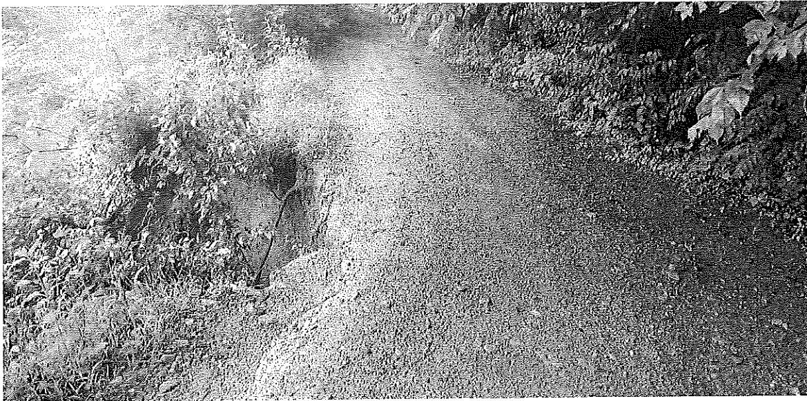
Dick's Creek Erosion – near STA 314+75
